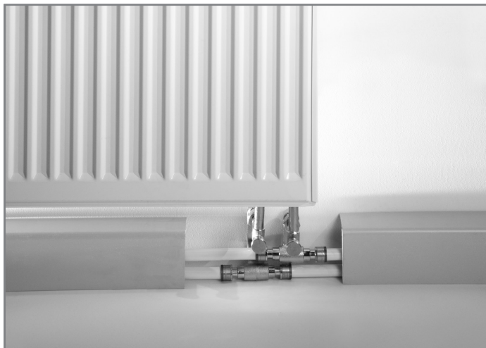
Radiator connection from the skirting board
