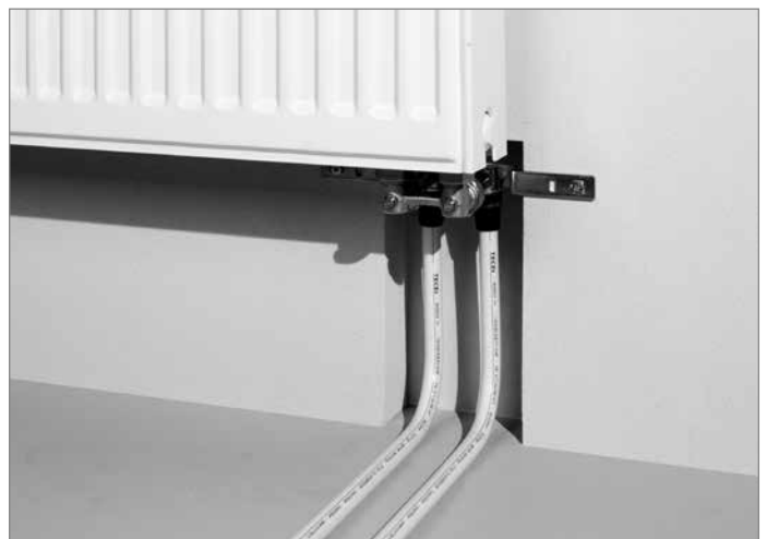
Radiator connection with radiator mounting unit, wall-mounting - connected to the valve block
