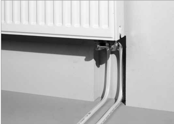
Radiator connection from the wall
