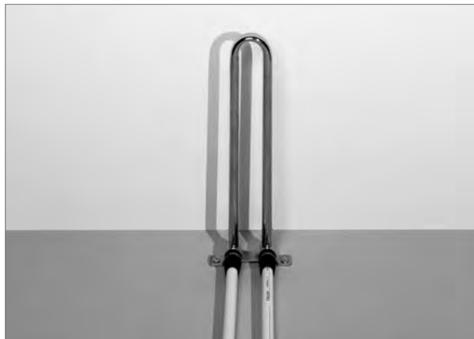
Radiator connection with radiator mounting unit, floor-mounted – ready for pressure test
