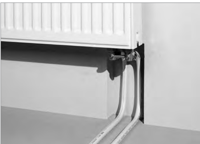
Connection of radiator to pipe coming out of the wall
