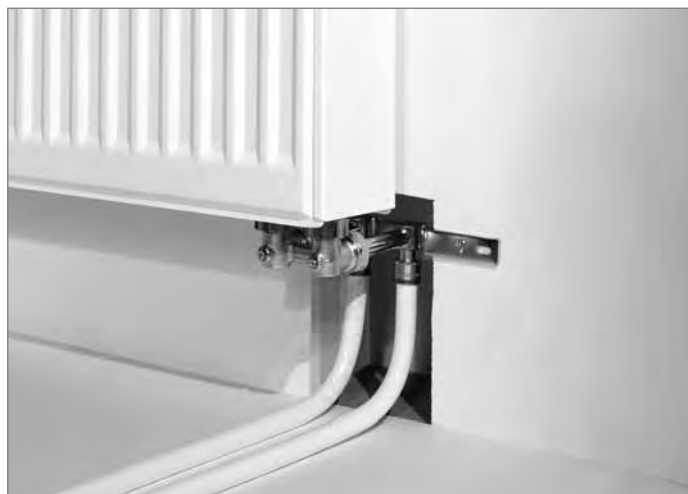
Radiator connection using radiator mounting unit – connected up to the valve block
