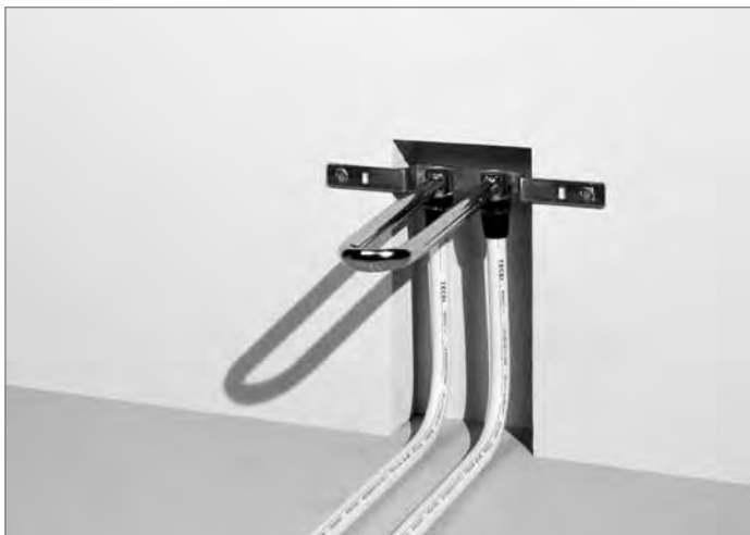
Radiator connection with radiator mounting unit, wall-mounted – ready for pressure test
