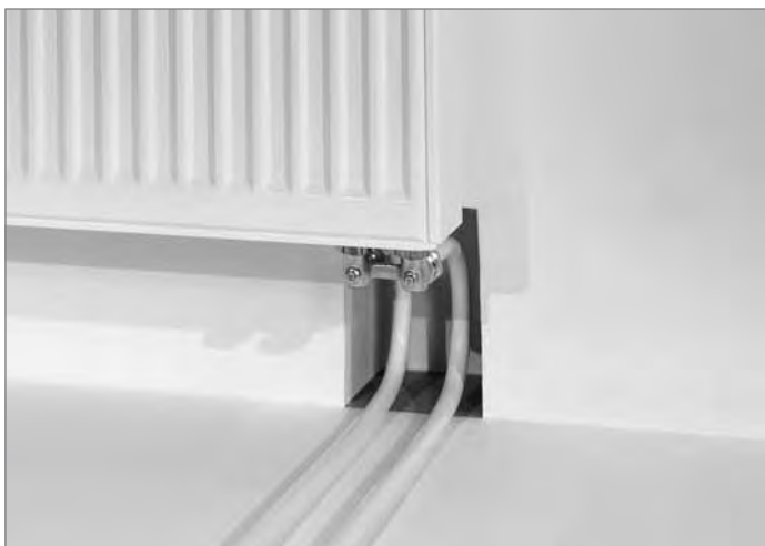
Connection of radiator to pipe exiting from the wall
