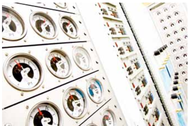
System for checking the creep rupture strength of installation pipes.
